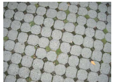
“SPECIAL” PAVING CAN HELP TO VISUALLY DISTINGUISH KEY STREETS WITHIN THE PLANNING AREA, AND CAN SERVE AS A TRAFFIC-CALMING DEVICE. PERMEABLE PAVERS (BOTTOM) ACCOMPLISHES THESE GOALS WHILE HELPING TO MANAGE STORMWATER RUNOFF
